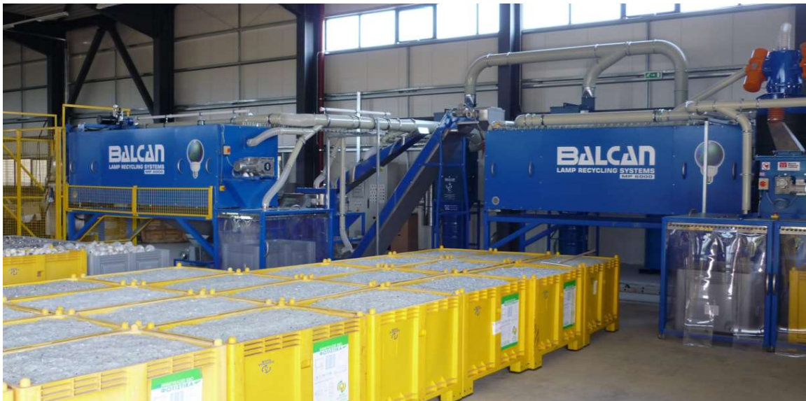
Figure 2. Fluorescent lamp recycling unit
