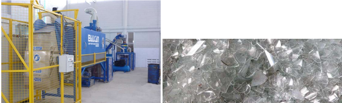
Figure 3. CFL recycling unit fitted in Surabaya Indonesia 2013 and glass cullet from the process.
