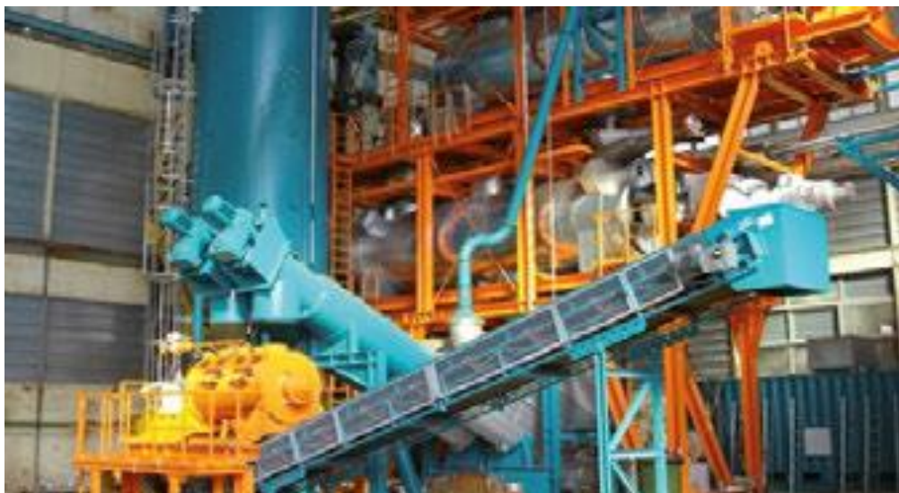
Picture 15. Indirectly heated Vacuum Distillation unit. (Source: econ industries GmbH cited in UNEP/ISWA 2015)
