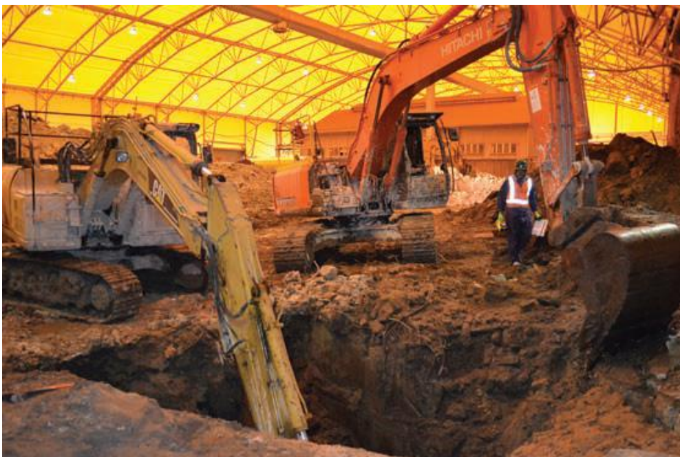
Picture 8: Interior of Odour Control Enclosure during excavation Source: Australian Federal Government (2013)
